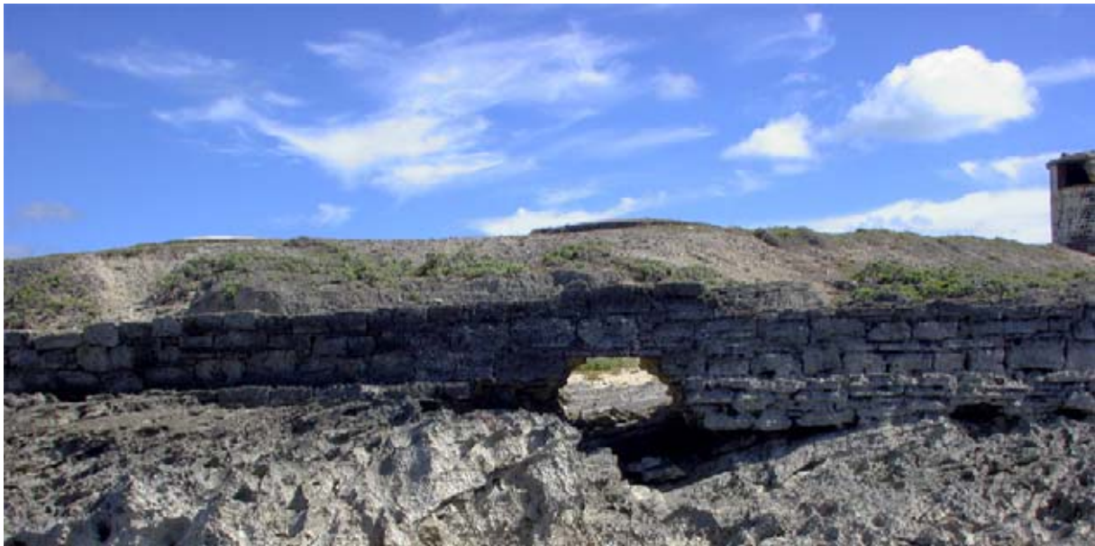
The outer face of the Lower Battery Wall A 3, showing the need for repair, with the Upper Battery behind. (02jv1822)
