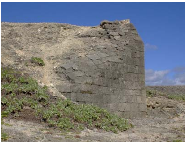
The South-East Wall and Rampart of the Upper Battery showing the stone cut to fit the different angles and the capping of the wall tops. (02jv1620)
