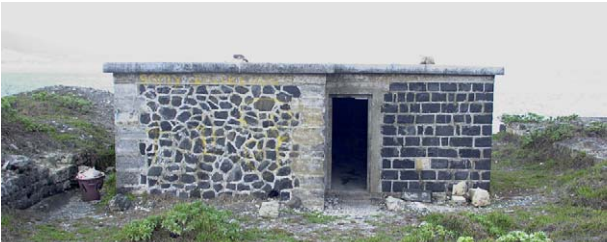
The west side of the Central Building showing the earlier walling on the right and the addition on the left with pre-cast cement blocks used as quoins, and the uncoursed masonry style. The entire building was given a ring beam and new roof and the earlier doorframe was revamped. (02jv0402)
