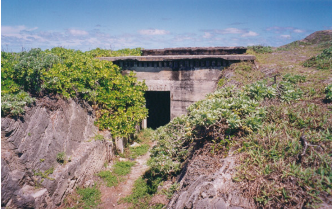
The Rock-Cut Feature looking towards the entrance to the Underground Generator Halls. The rock-cut channel at the top on either side is almost totally obscured by vegetation. (02cn0417)
