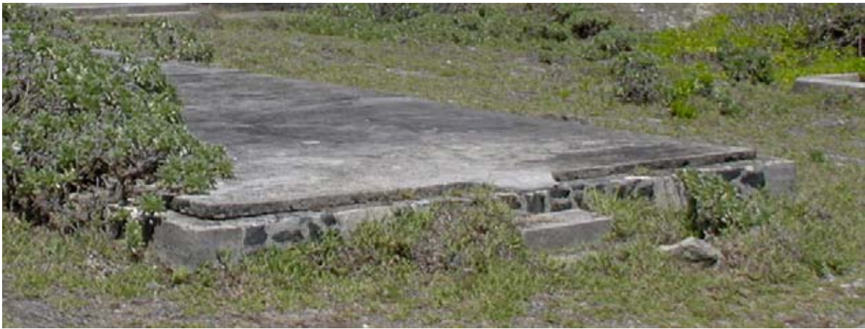
Pre-cast concrete blocks have been used at the corner of the building platform. (02jv2215)
