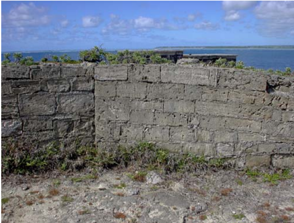
The vertical joint between Walls D1 and E. Note the difference in masonry styles and the change in the horizontal angle of the upper courses of Wall E. (02jv1911)
