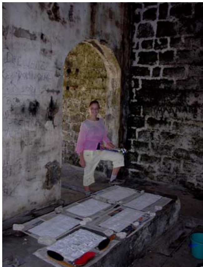
Squeezes drying on one of the generator plinths. One of the cable ducts runs through the door. (02jv0809)
