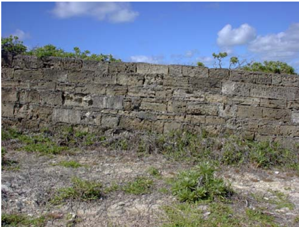
The inner face of part of Wall E showing how the courses of stone run parallel to the slope of the ground. Some of the graffiti from the 1840s are visible. (02jv1916)
