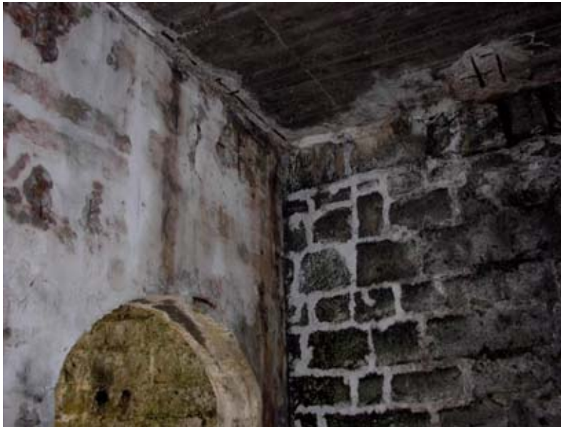
The Storehouse Generator Building showing the southern reinforced concrete partition with the arched door and the roof, both added in WW II. (02jv0810)
