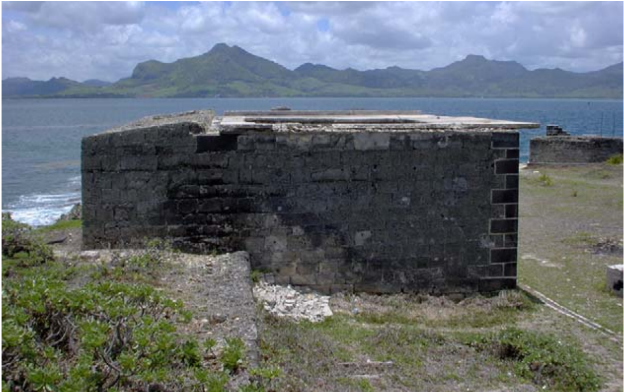
South side of the Storehouse showing the roof drain, the blocked vent and Wall E with the berm on the left. Part of the broken WW II roof has been piled in the corner to limit further damage from fires. The drain at right is WW II. (02jv0121)
