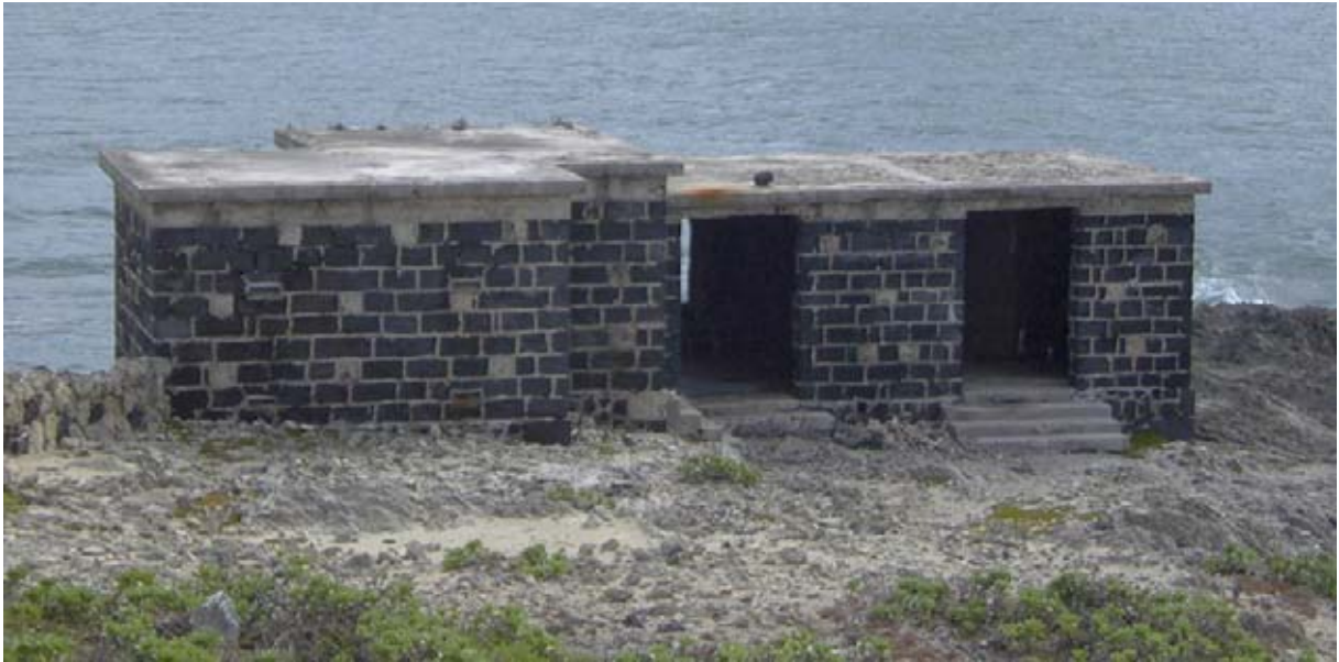
The Western, Searchlight, Building - Structure 12. Note the pattern of pre-cast concrete tie blocks and the keystones over each of the vents in the original structure. In WW II a ring beam, reinforced concrete roof, concrete steps and a new floor containing ducts for electrical wires were added. The walling was repointed and the openings on the seaward side were greatly reduced. (02jv0419)
