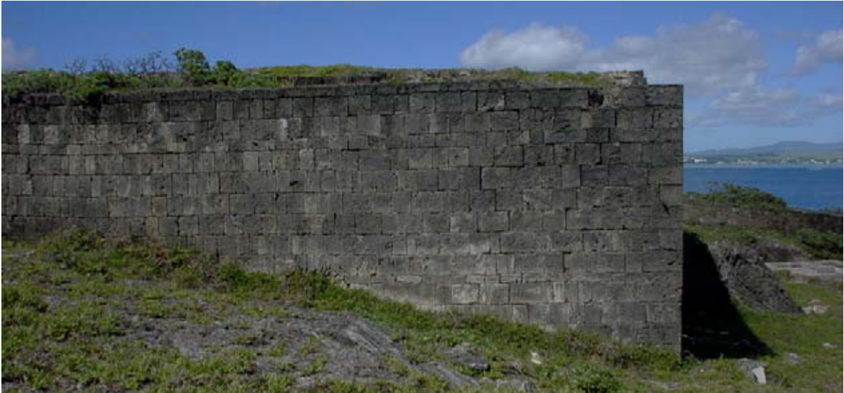
The Terrace Wall of the Upper Battery showing the corner with the North Wall. (02jv2003)
