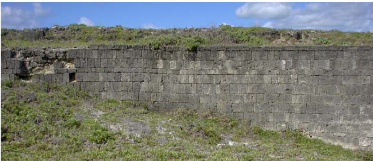
The central section of the northern stretch of Terrace Wall. The Battery Wall and Cannon Emplacements are above. (02jv2004).
