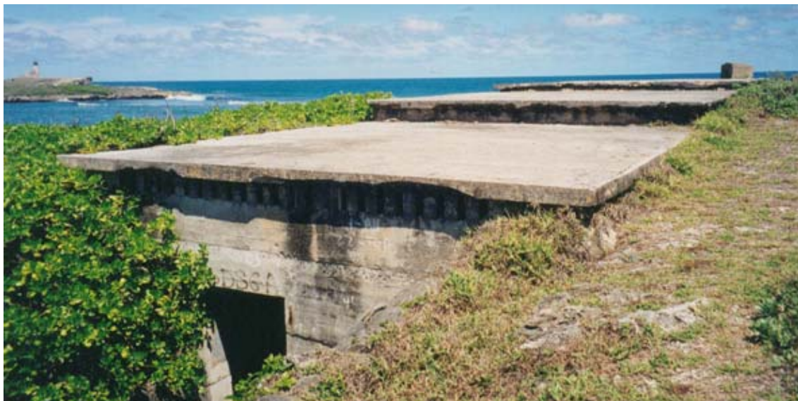
The Underground Generator Halls, Structure 7. The ventilation grills can be seen in the shadow of the roof. (02cn0415)
