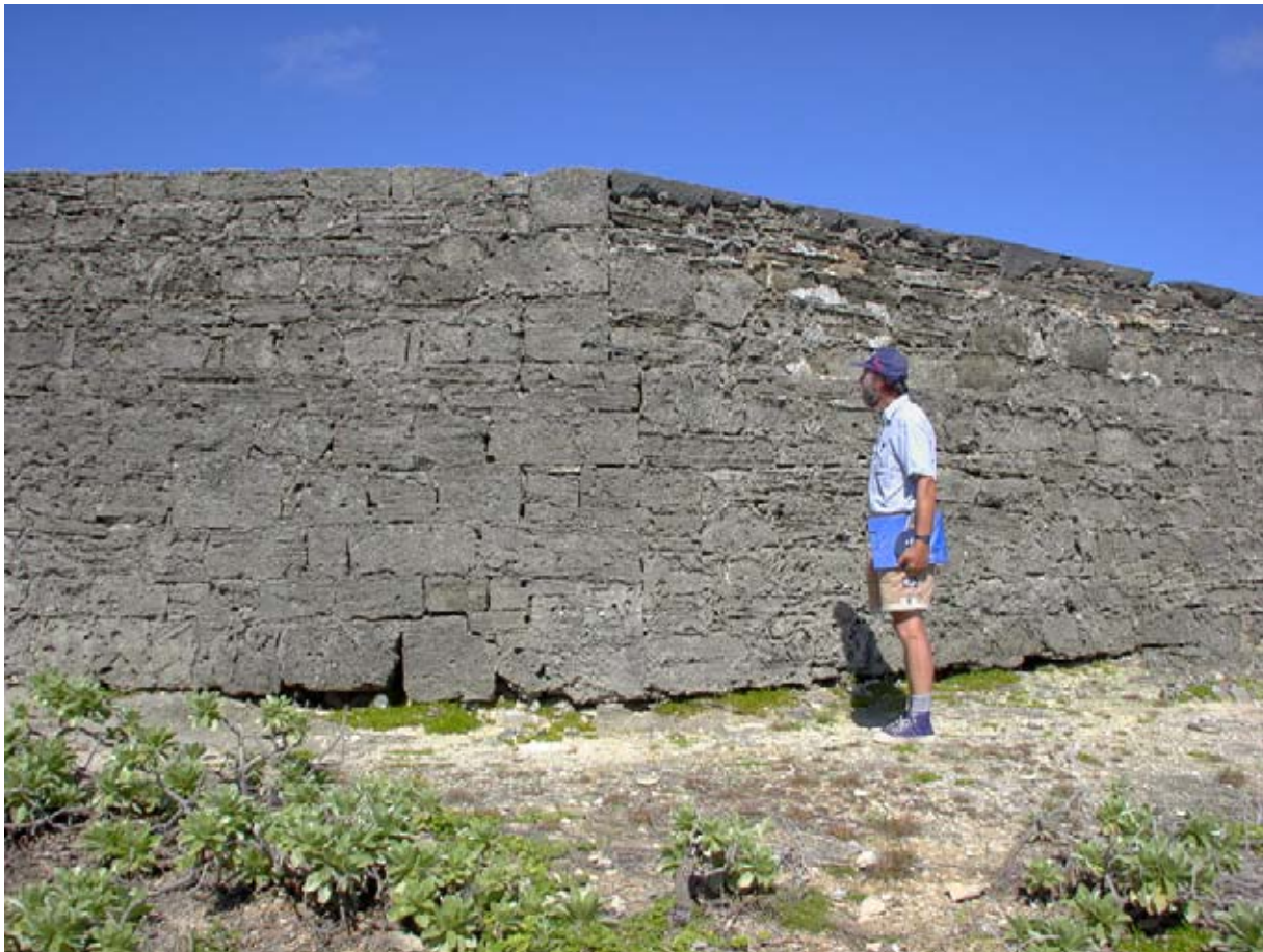
The junction of the main wall of the Lower Battery, Wall A at left, and Wall B showing the butt joint, broken by the insertion of the fourth stone from the bottom, and the offsets. (02jv1807)
