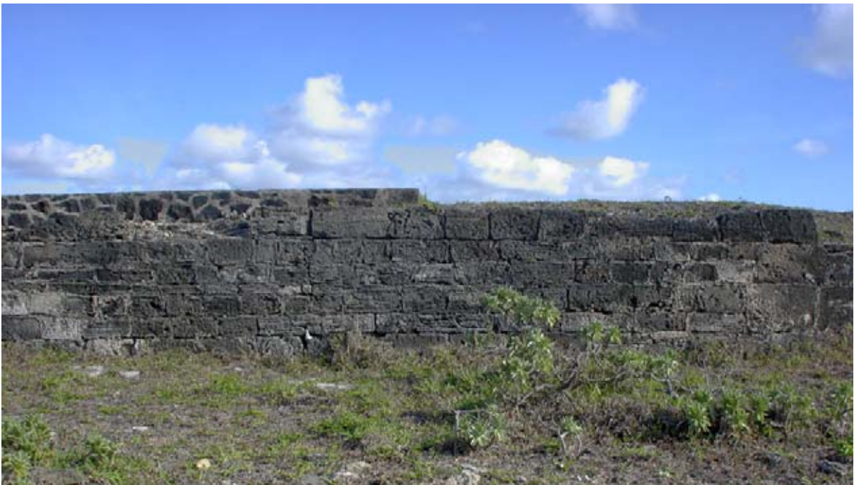
Wall H with WW II Structure 22 on top. The top edge of the uppermost row of stones is chamfered. (02jv18)
