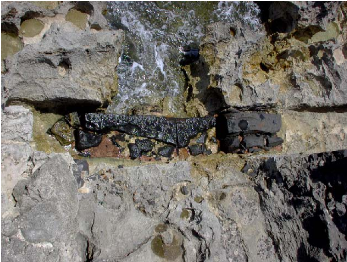
At high tide the buttress in front of Wall F is washed by the sea. (02jv1211)
