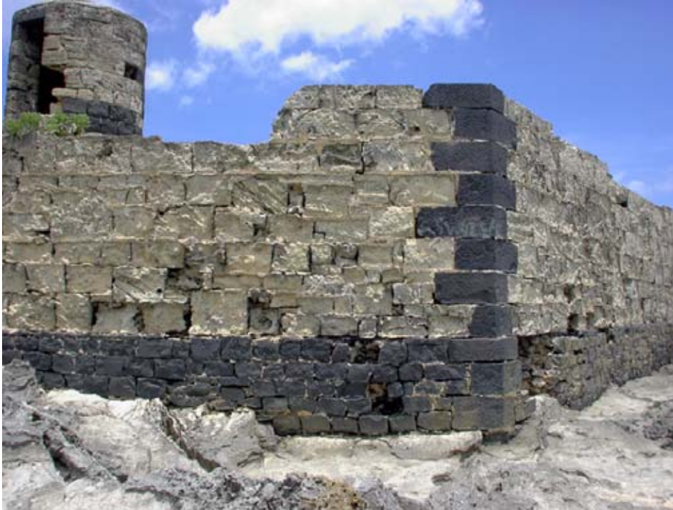
The corner of Wall F3 and F4 showing the need for repair and erosion of the coral blocks. Immediately in front of the footings is the rock-cut trench that once contained the additional basalt of the external buttress. The North-West Sentry Post stands above. (02dpjv0216)
