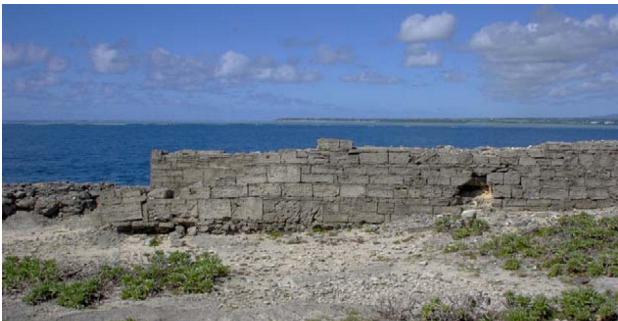
Wall D3, with Wall A behind. The large block at the base of the southern end of Wall D3 has been reused from an earlier cannon emplacement. (02jv1906)
