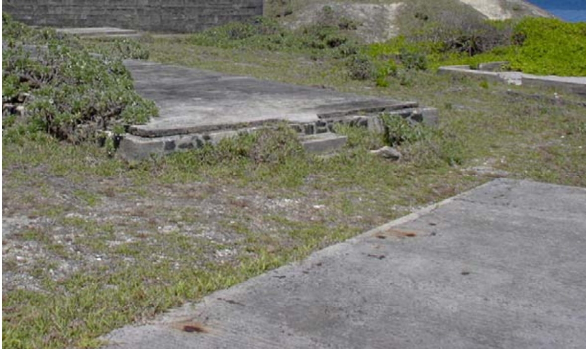
Rusty remains of iron pins can be identified on some of the structures. Most of the building platforms were made of uncoursed basalt with precast concrete corner blocks. (02jv2215)
