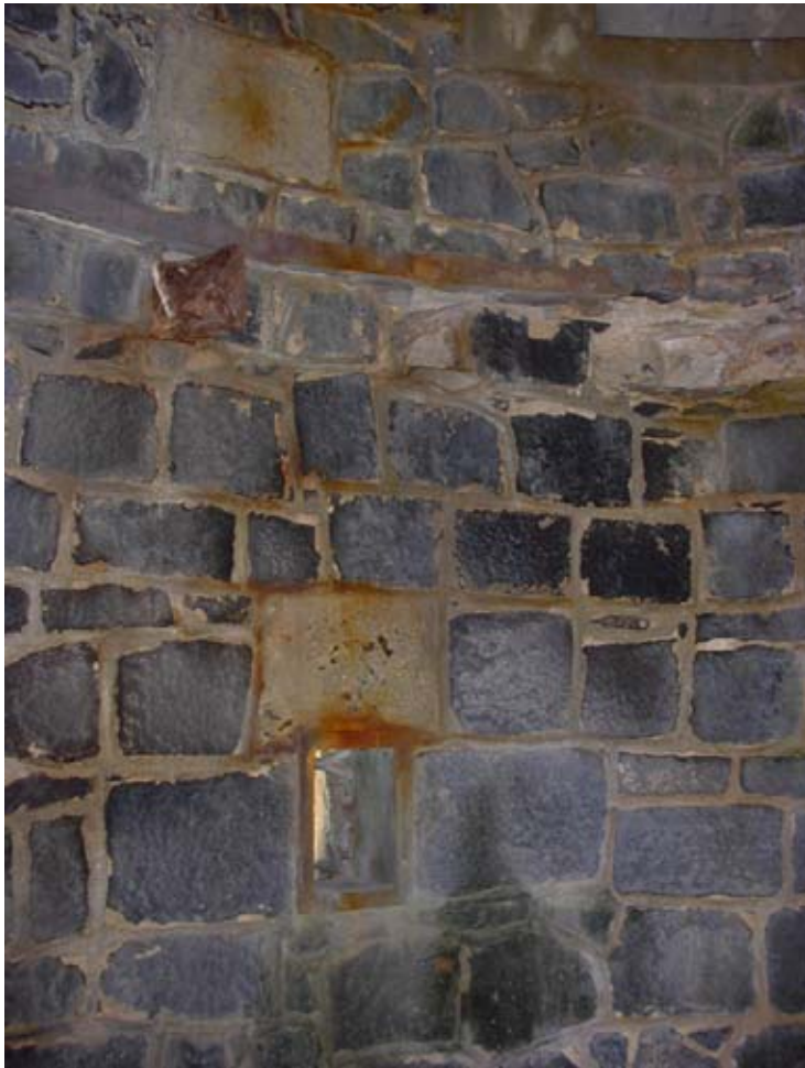
Inside: a vent capped by a pre-cast concrete tie block and flanked by shaped stones. The cement rendering formed a skirting above the timber floorboards. (01jv0920)
