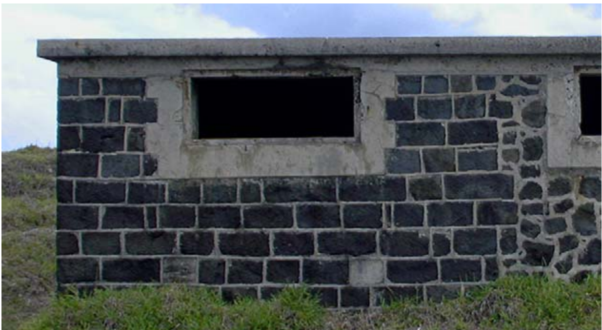
Basalt ashlar and concrete tie blocks characterise the first building phase of the Central Building. The concrete window surround is WW II. (02jv0204)
