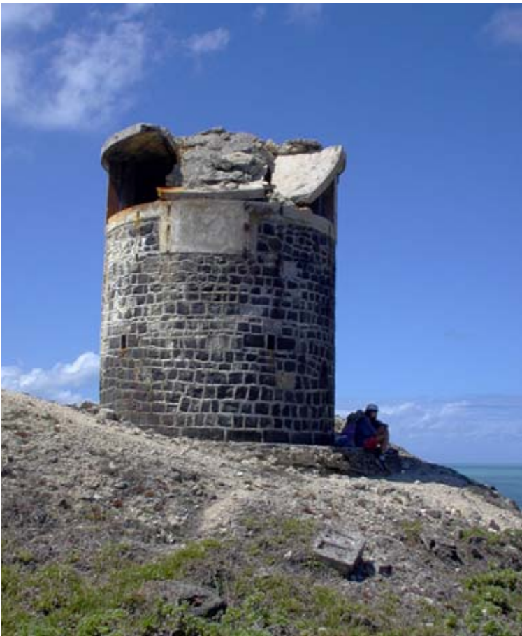
The bottom course of large shaped basalt blocks sits directly on the concrete base. Large shaped stones also flank the vents. The WW II roof has collapsed. (02vj0913)
