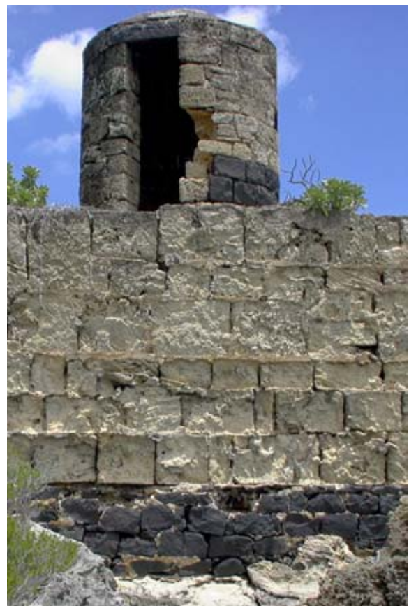
The North-West Sentry Post, at left, atop the defences, showing recent damage to the door. (02jv0217)
