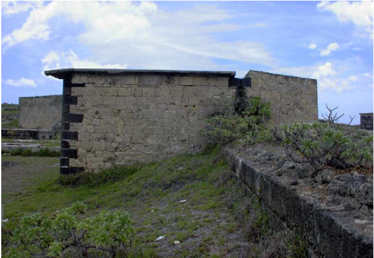
The south side of the Storehouse, Wall F5 and the internal bank. Note the roof drain, the blocked vent and the sloping top of the casemate. (02jv011).
