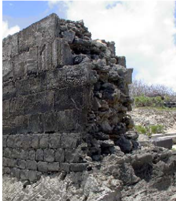
Wall F showing the external basalt footings founded directly on the irregular bedrock and the layered rubble construction of the wall core. (02jv0208)
