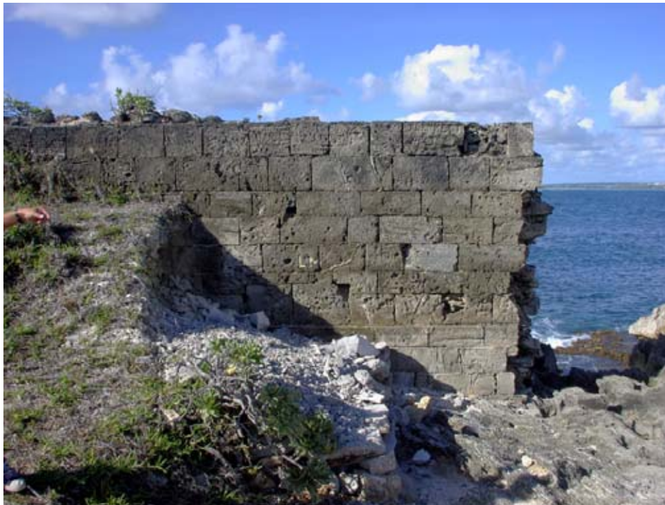
The south side of the breach in Wall F showing the offset and the urgent need for consolidation. The inner Bank and Berm has now afforded some protection by the piling up of concrete debris from demolition of the Storehouse roof. (02jv1001)
