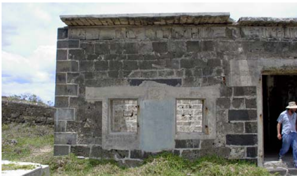
Two new windows replaced single opening which is indicated by the surviving basalt lintel and sill. The door was also remodelled with a concrete lintel and sides. (02jv0115)
