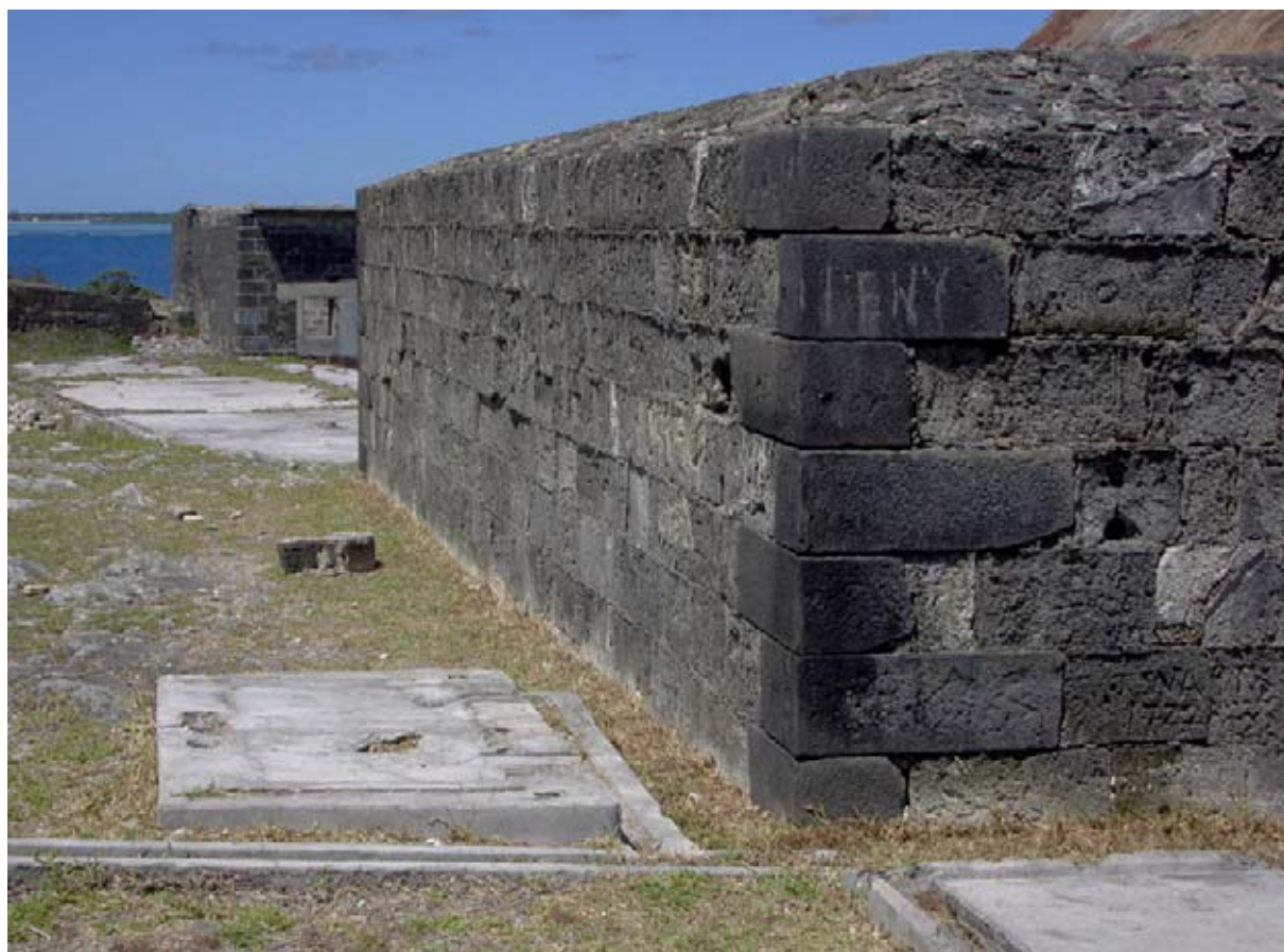
The Showers, Structure 25, and drain, at the south-east corner of the Powder House Enclosure Wall. Part of Structure 26 is at right. (02jv2208)
