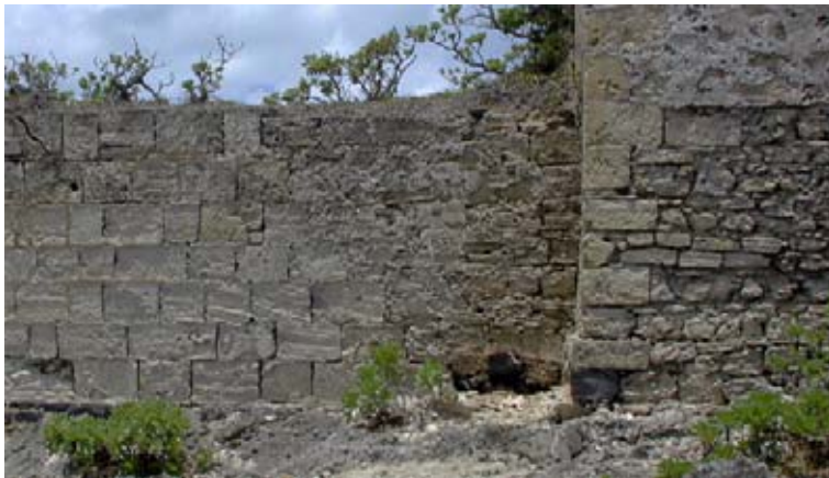
Wall F5 at left showing the rebuilding and extension, with a drain at the base, in a very different style. The upper part of the rear wall of the Storehouse, at right, shows how the face was rendered with lime mortar above the top of the now vanished bank which once protected the lower part. (02jv0201)
