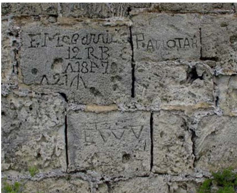
Graffiti on the seaward face of Wall F2. Digital photography with a high resolution camera will produce excellent images that can be enhanced on screen or used to make good prints. Production of scale drawings will require time and patience, but need not be done during the short field season. (02jv0222)
