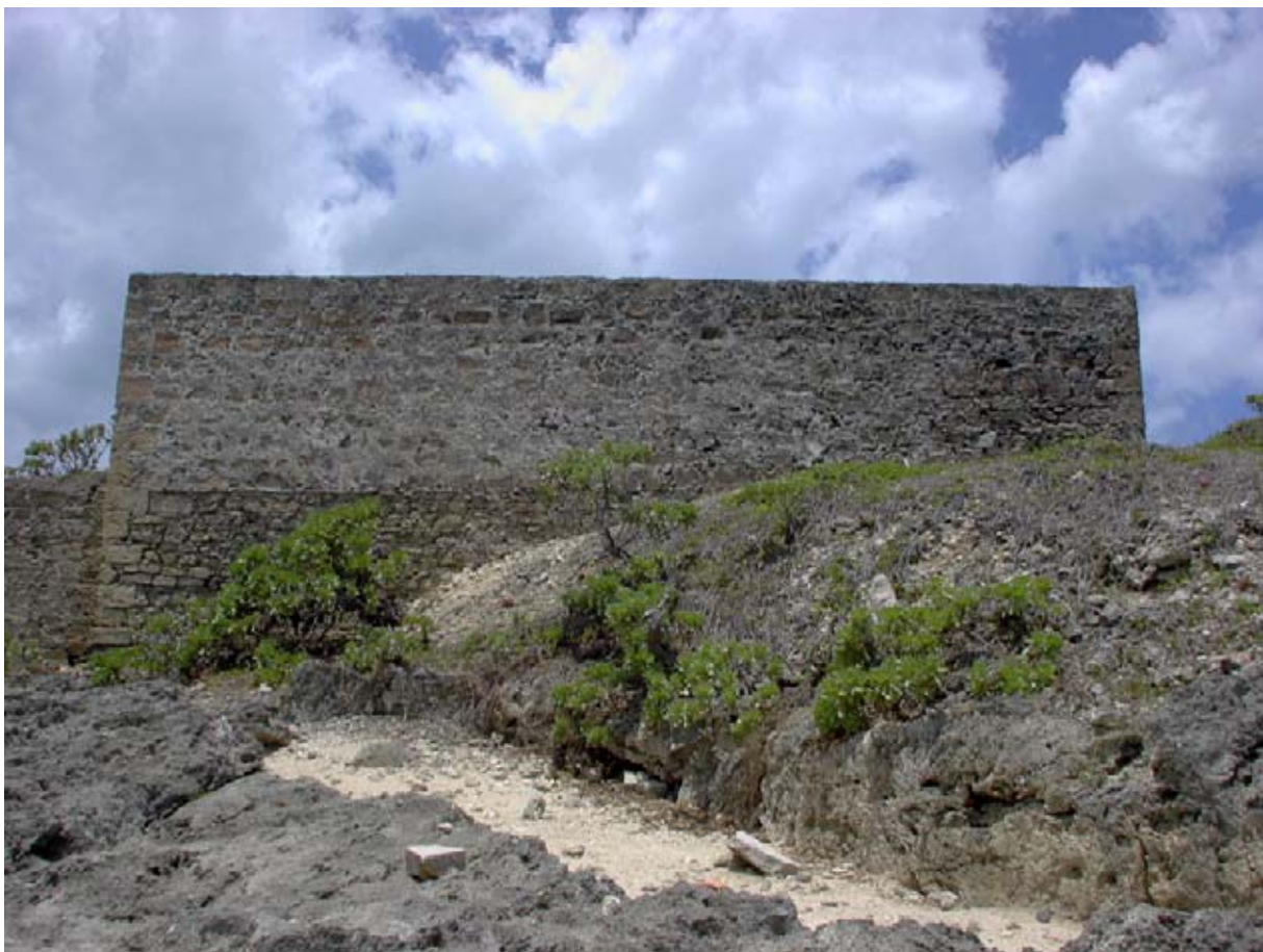
The rear of the Storehouse. The terrace wall retaining the foundation was protected by a bank and berm which has washed away below the rendering on the left. (02jv012).
