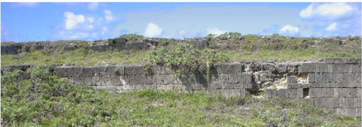
An extension of the picture above showing the need for repair. (02jv2005)
