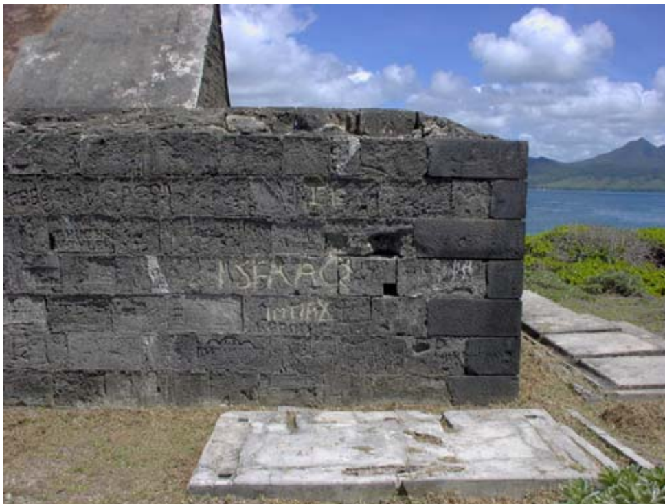
The slanting top of the enclosure wall was levelled in order to seat water tanks for the WWII showers. (02jv1111)
