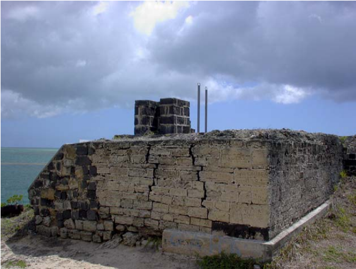
The need for repair. (02jv0110)
