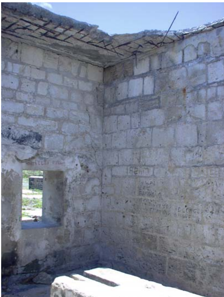
Most of the concrete roof has been removed in the southern room of the Storehouse. (02jv0811)
