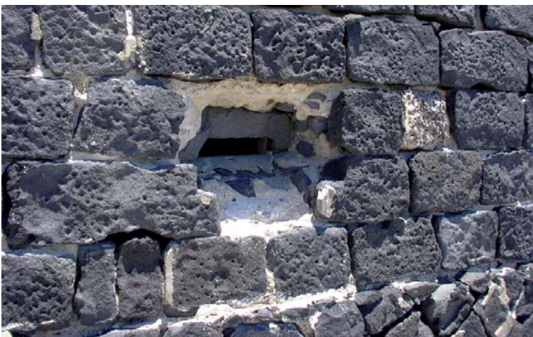
A broken vent reveals construction details.
