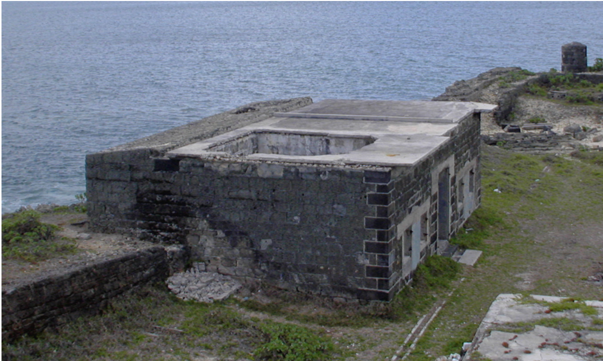
The Storehouse as seen from the Upper Battery showing the broken concrete roof. (02JV0308)
