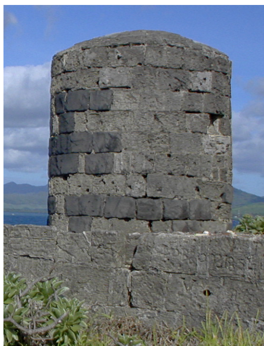
Rear view of North-West Sentry Post showing one of the small windows. The random mixture of coral and basalt blocks is to be noted.
