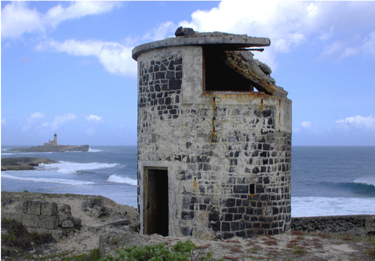
The Observation Tower with its partially collapsed roof. (02jv0401)
