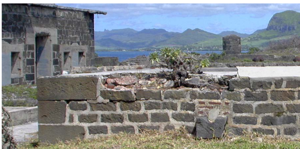
South-west corner of the cistern where blocks from the uppermost course should be replaced and vegetation carefully removed. The blocked basalt 'spout' shows a red brick blockage with a circular hole perhaps allowing for a pipe and later blocked by a cement mortar. (02jv2107)
