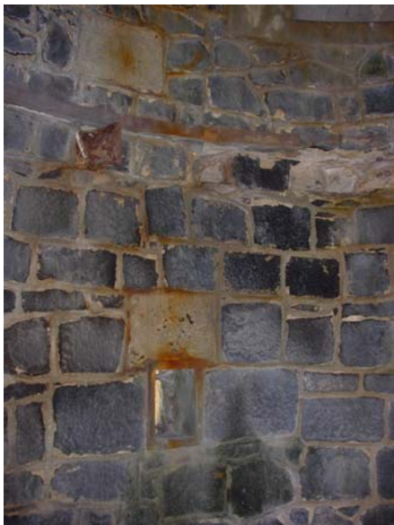
Concrete tie block over vent with traces of first floor timbers above. (02jv0920)
