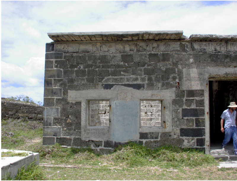
Digital photograph of part of the front elevation of the Storehouse. (02jv0115)
