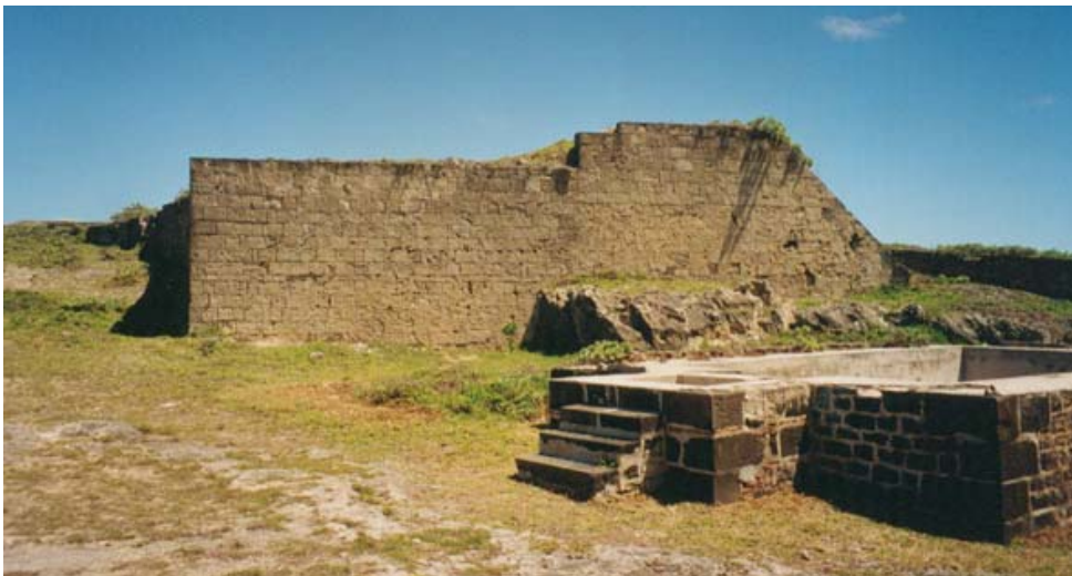
The early rock-cutting partially beneath the north wall of the Upper Battery. (02cn0431)
