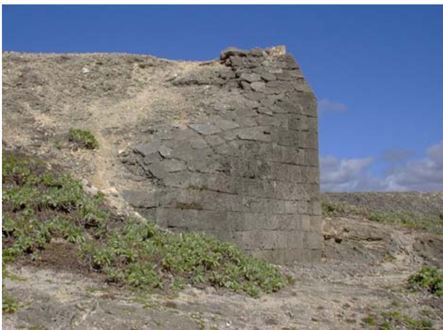
The southern end of the Upper Battery showing erosion caused by the track down the rampart, the deterrent effect of bushes and the inert path at the base of the wall. (02jv1620)
