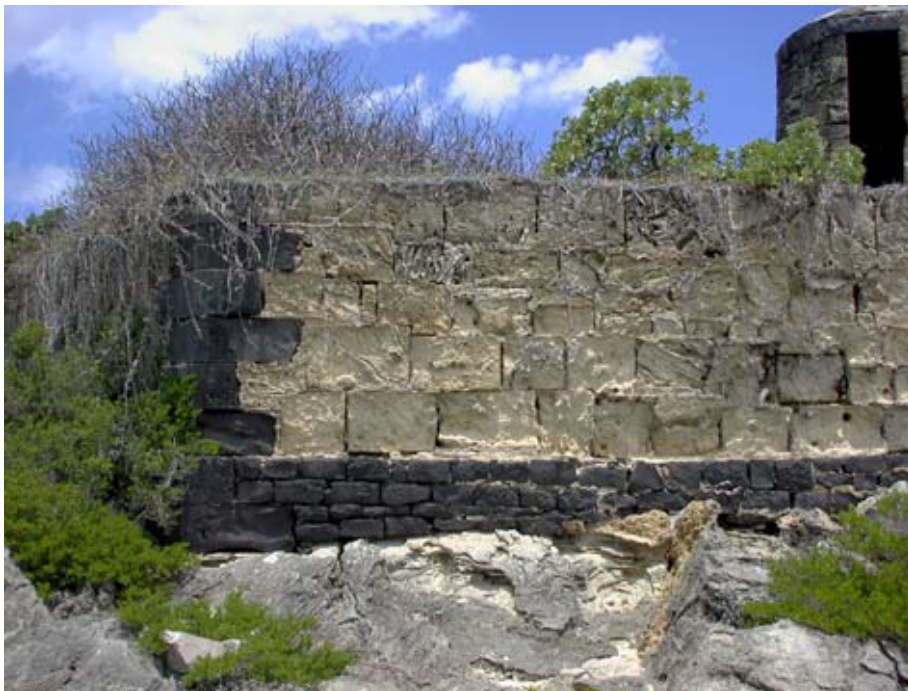
Vegetation on the wall top prevents visitors walking along the wall edge and dislodging stones. Note how the soft fossilised coral is slowly eroding. (02jv0218)
