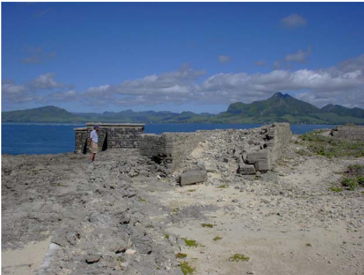
Wall A and Wall D with the rubble fill showing the way in foot traffic and nature are eroding the ramped casemate fill and has undermined the base of the wall on the right. (02jv1903)
