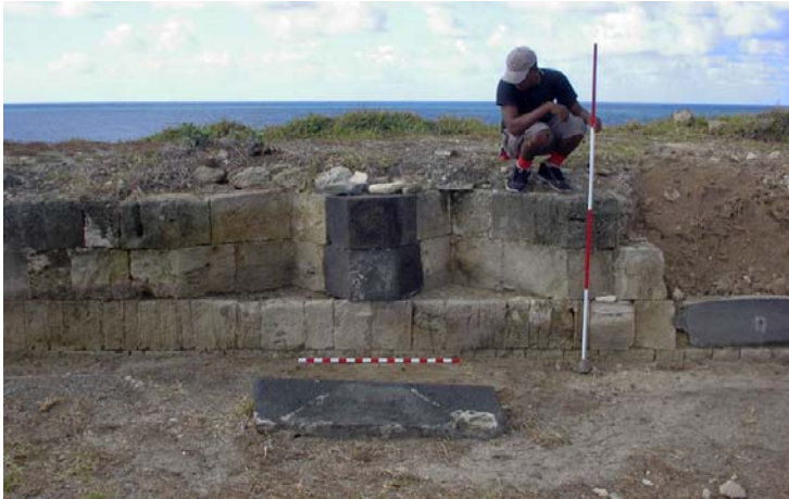
Some of the basalt stones were put back in place and where necessary a lime mortar, similar to the original one, was used. (03jv3510)
