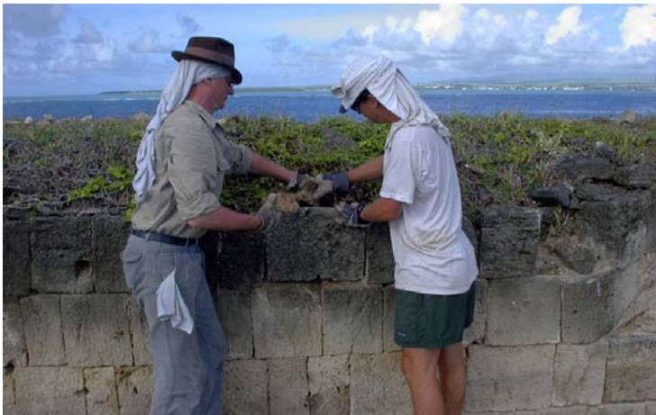
Conservation First Aid... Bradley and Jonathan pushing back into position the displaced stone seen at center left in the previous photo. (03jv1304)
