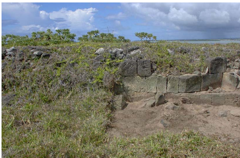
Full documentation can only be carried out after vegetation, rubbish and blown in sand has been cleared from in the front of the structures. (03jv0217)
