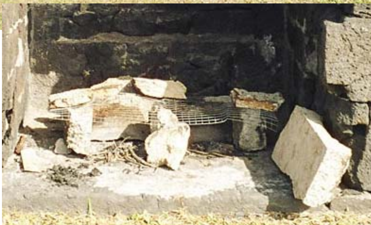
Figure 9: Barbecues lit inside the hot shot furnace seriously endanger the already damaged structure. (03cn0207)
