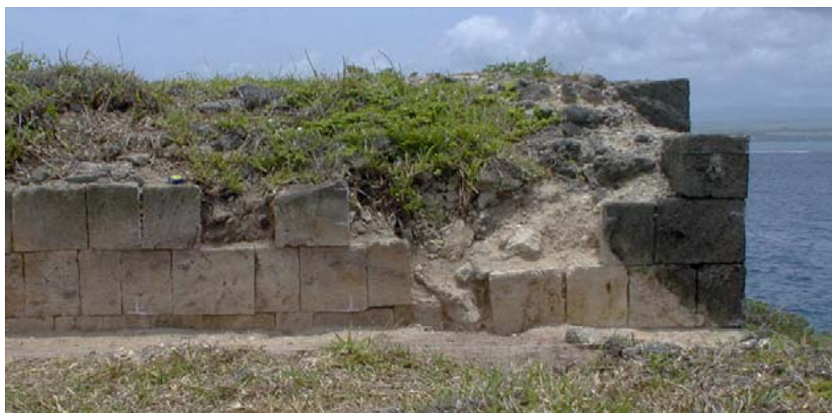
Figure 21: After clearance it was evident that the Parapet Wall of the Upper Battery was not bonded to the North Wall. (03jv1101)
