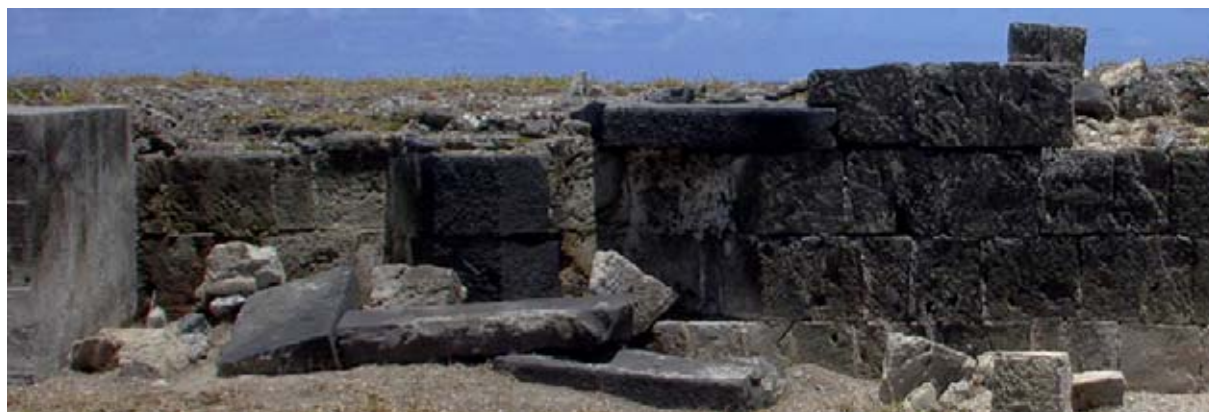
Figure 23: On the right side Emplacement 5 the fifth course comprises basalt lintels locked in place by coral blocks cut to fit. (03jv0603)
