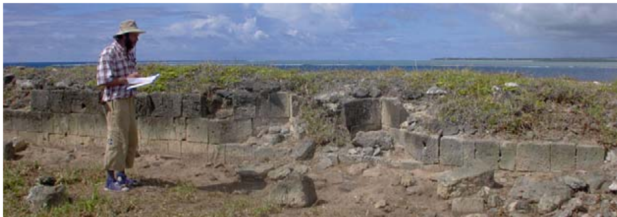
Figure 22: The stretch of Parapet Wall either side of Emplacement 1 has regular courses and staggered vertical jointing, although there is no bonding pattern. (03jv0208)
