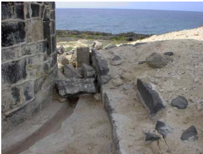
Figure B: Displaced basalt blocks, the basalt retaining wall and the eroded bank on the north-west side of the Observation Tower. (03jv0915)
