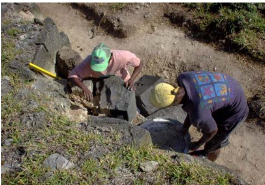
Figure 11: Basalt blocks fallen from the emplacements were set back in their original position. (03jv1610)
