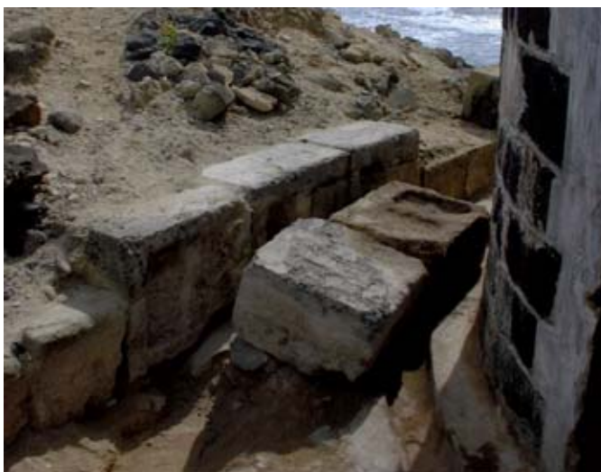
Figure C: World War II precast hollow concrete blocks were used to retain the bank on the north-east side of the Observation Tower. The two fallen blocks seen here, together with others now lying at the foot of the bank, could be put back on the retaining wall. (03jv0913)
