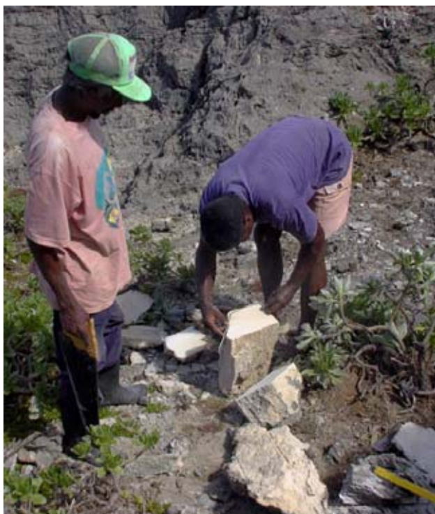
Figure 15: New blocks of coral were cut from the quarry and shaped to replace missing ones. (03jv1716)
