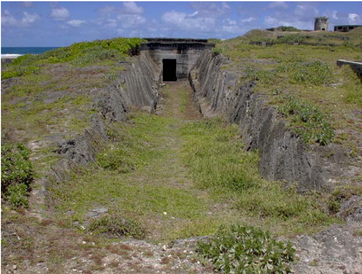
Figure 40: The Underground Generator Halls and the Ditch were cleaned and vegetation was cut back. (03jv2908)
