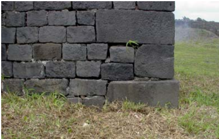
Figure 56. Replacement of the stone has restored the stability of the bottom course of masonry. (04jv1216)
