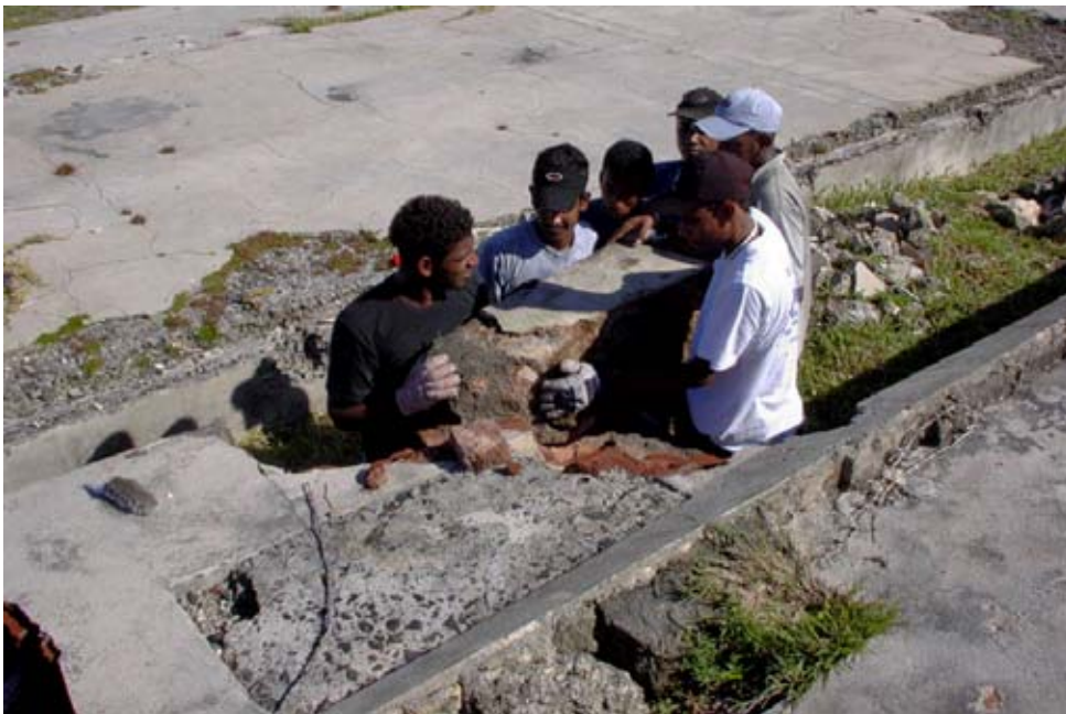
Figure 21. The workmen uniting efforts to put back a large basalt block dislodged from the settling tank of the Cistern. (04jv0905)
