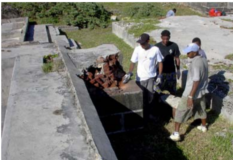
Figure 57. A large basalt corner block was put back on the settling tank of the Cistern. (04jv0903)
