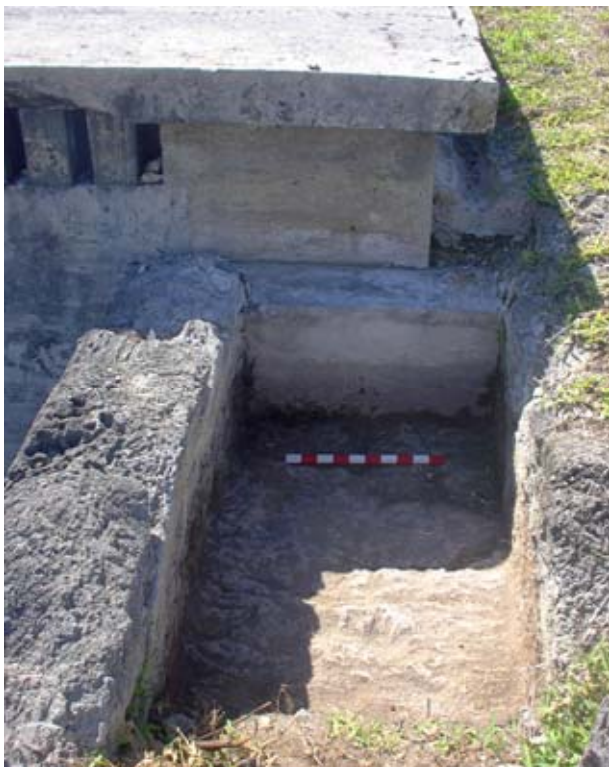
Figure 50. Trench TR14 showing the channel blocked by the front wall of the WW II Generator Hall. (04jv1517)
