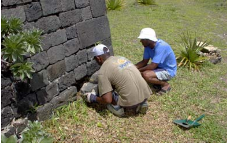
Figure 55. A stone that slipped from the base of the Hot Shot Furnace was put back in its place. (04jv1213)
