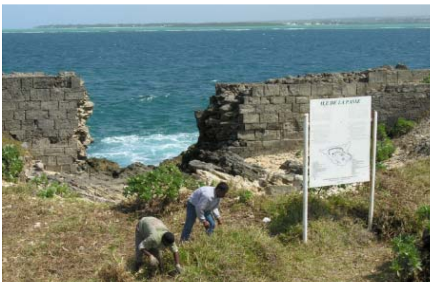
Figure 8. Workmen were employed to clean up the islet, clear vegetation and help with heavy excavation work and backfilling. (mp05nc1209)
