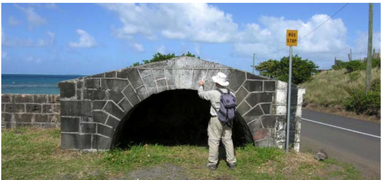
Figure 33. The vault at the southern end of the battery was documented with the help of digital photos and control points for photo-rectification. (md05nc0101)
