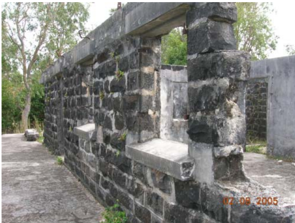
Figure 31. Roofless masonry building. (md05nn0148)
