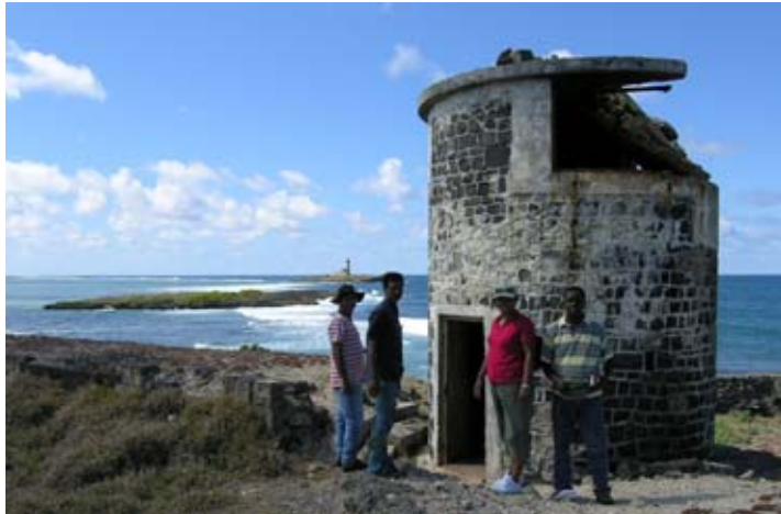
Figure 32. The Observation Tower with its dangerous collapsed roof. (mp06nc1311)
