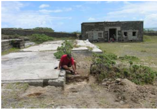
Figure 12. Trench TR19 located over the north east corner of the WW II platform, Structure 18. (mp06nc0642)
