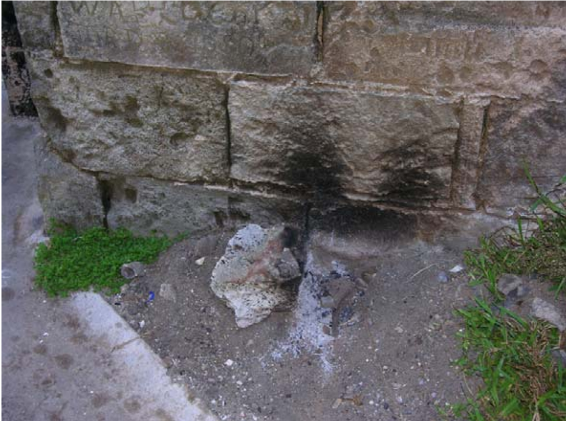
Figure 5. Heat from the barbecues set up next to the walls damage the fossilized sand blocks.
