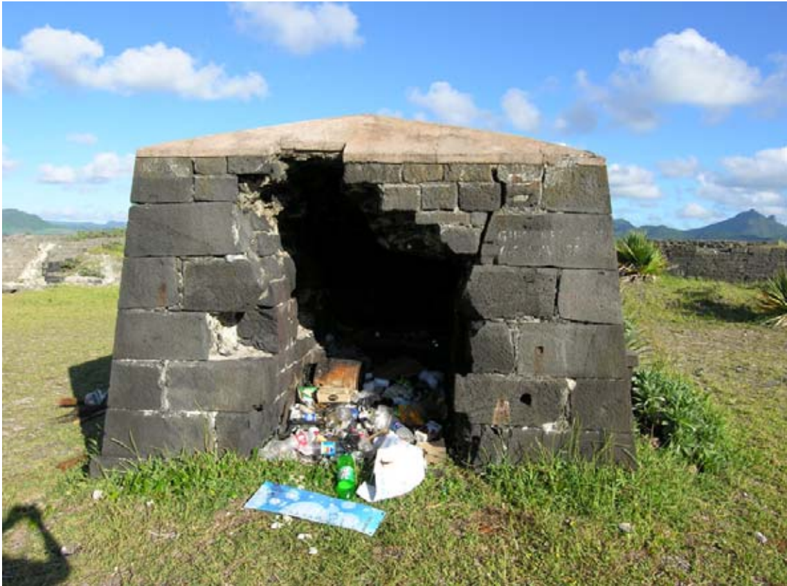
Figure 4. Rubbish left in the Hot Shot Furnace.
